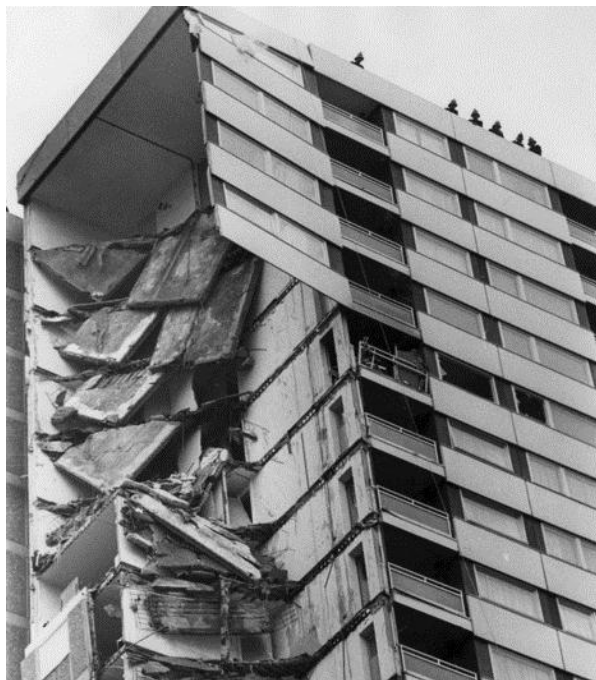
Figure 1 Collapse of Ronan Point [12]
