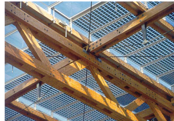
solar modules integrated into the glass skin
