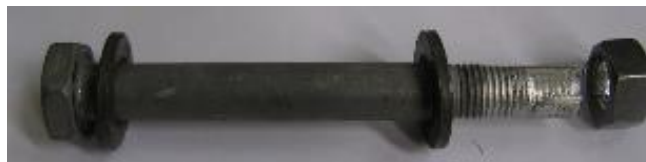
Stripping of bolt threads
