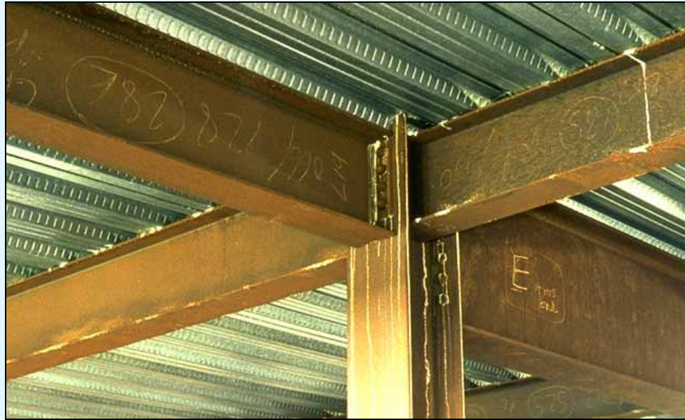
Figure 1.2 View of unprotected steel structure
