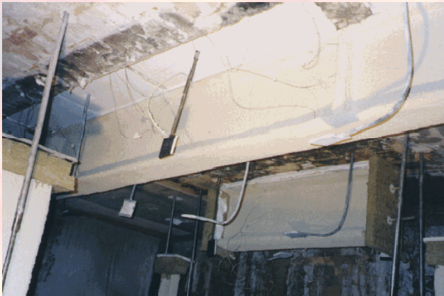
beam before fire test
