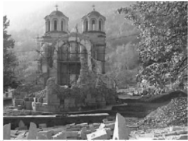
Figure 5. Damage to the vault in the narthex.
