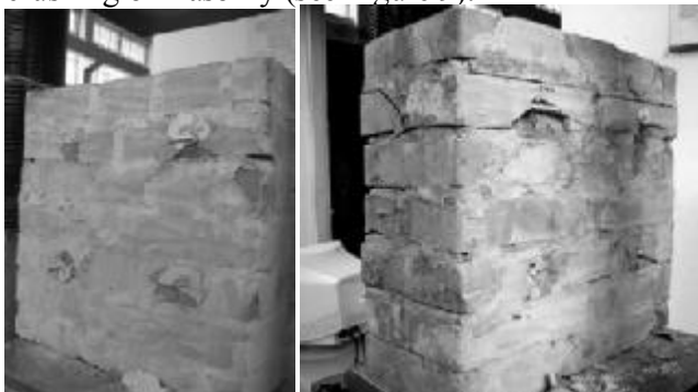
Figure 9. Failure modes for chemical anchor connections a) \phi 8 diameter and b) \phi 10
