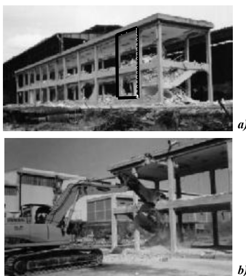
Figure 11. The original RC building after the partition removal (a) and subdivision in separate modules (b).
