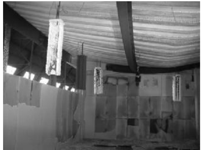
Figure 1. Compartment after the seventh large Cardington test, see (Wald et al, 2006), the slab residual deformation 915 mm.
