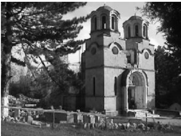
Figure 4. Damage to the belfries, northwest view.
