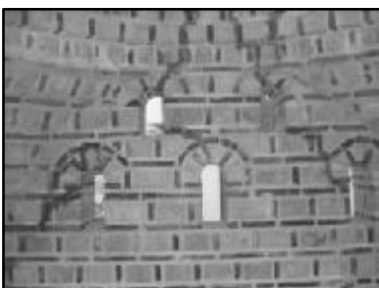
Figure 10. Damage of the mosque, interior
