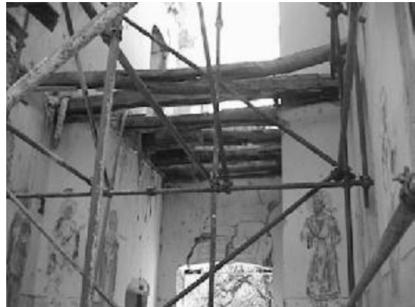
Figure 6. Damage to the floor structure.
