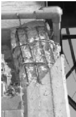
(a) Damaged end column
