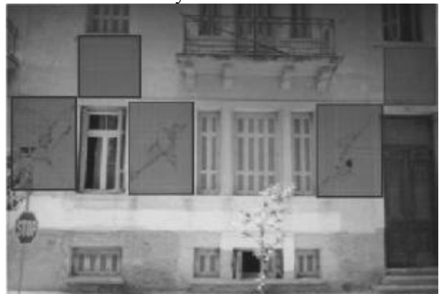
Figure 4. Weak area on masonry façade and location of metal sheeting (SP) or steel wire mesh (WM)
