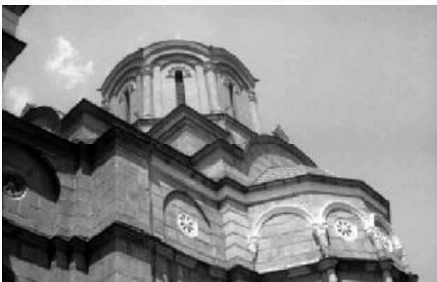
Figure 16. View of the visible dilatation
