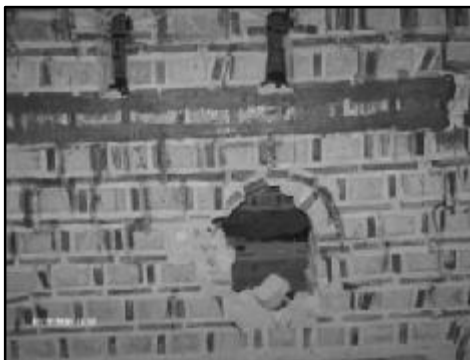
Figure 17. Details of damage, phase 3
