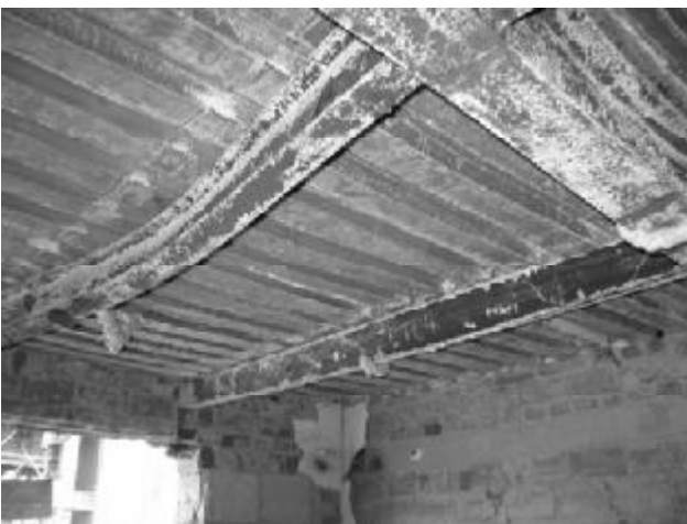
Figure 7. Beams after the compartment fire test.
