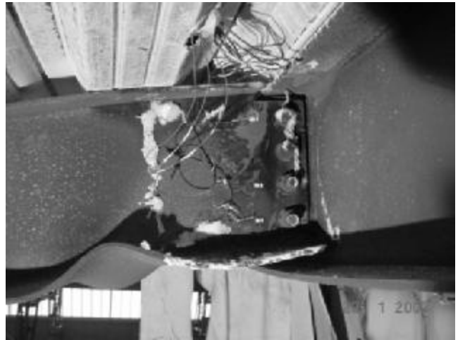
Figure 4. Deformation of the fin plate beam to column connection during the seventh large Cardington fire test, see (Wald et al, 2006).
