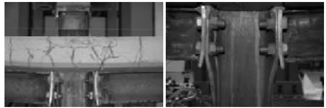
Figure 8. Collapse of the joint (sagging) under biaxial loading
