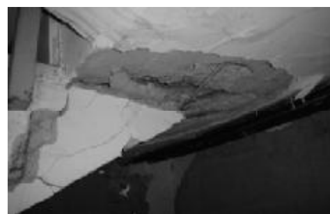
Figure 7. Damage to the staircase structure at the point of minimum lateral displacement (-12 cm in Figure 5).
