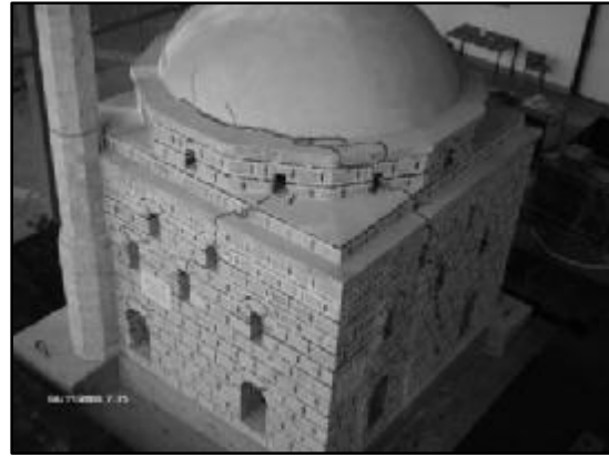
Figure 4. Damage of the minaret (horizontal crack) and of the mosque after phase 1
