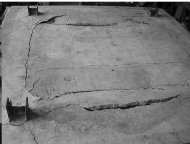
Fig. 7 Crack pattern of S3-FR
