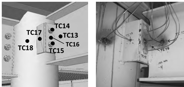
Fig. 2 Fire unprotected beam-to-column connection (B2-C2 to B2) in the 2 nd floor
