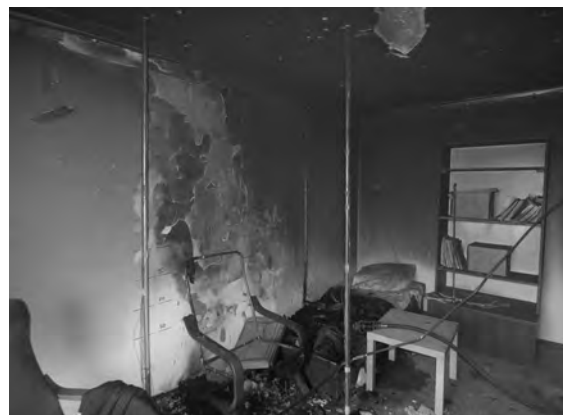
Fig. 4 Fire compartment after test no.1
