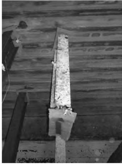
Fig. 2 Detail of surface of zinc coated member after fire
