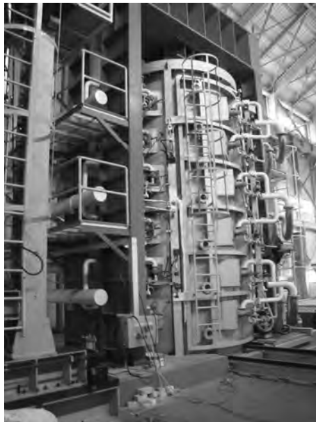
(a) 10,000 kN heating furnace
