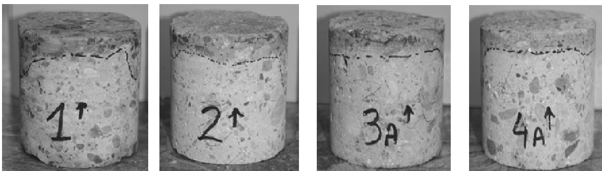
Fig. 4 Discoloration depth corresponding to the depth of destruction of the drilled concrete cores
