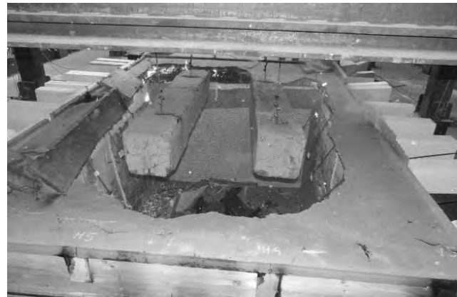
Fig. 3 Collapse of the composite slab
