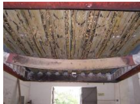
Fig.16. The deformation at the bottom of S-2 after the test
