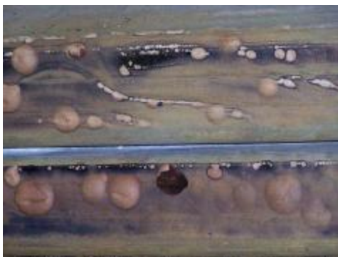
Fig.17. The steel deck after the test
