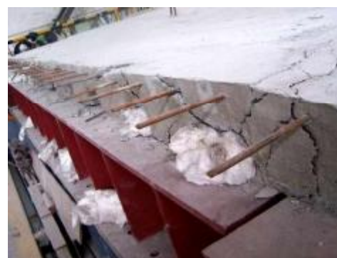
Fig.12. Cracks along the short side face
