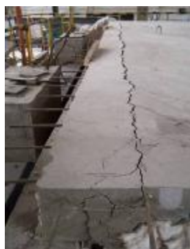
Fig.11. Cracks along the long edge
