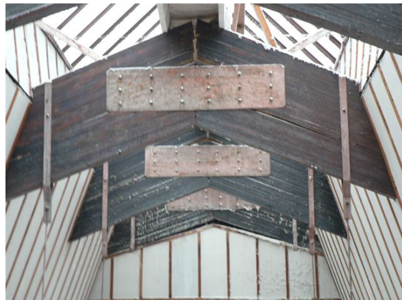
Fig.11 Assumed hinge in the middle of the roof frame, cracks on compressed heads of beams
