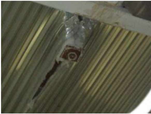
Fig.8 The broken ceiling, the ceiling hanger broke the aluminium sheet
