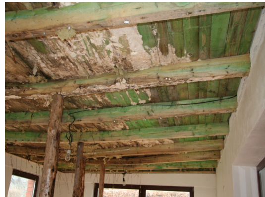
Fig.15 Timber roof system destroyed by the sponge colony
