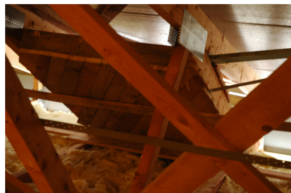
Fig.17 Additonal sytem of longitudinal global bracing that was not provided
