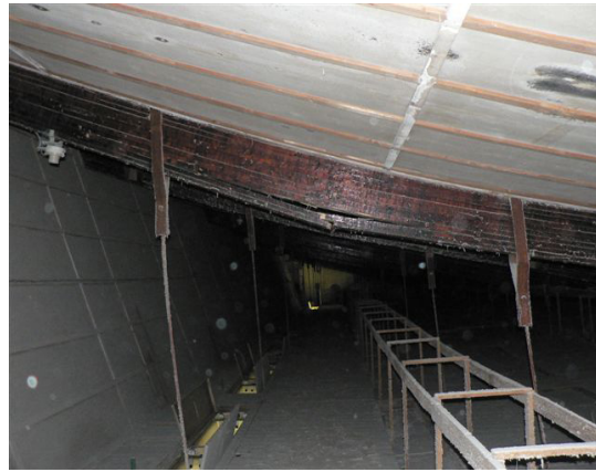
Fig.9 The deflected beam, rupture of lamellas, shear cracks
