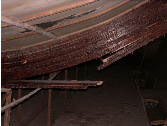
Fig.12 Final situation of beams before total collapse
