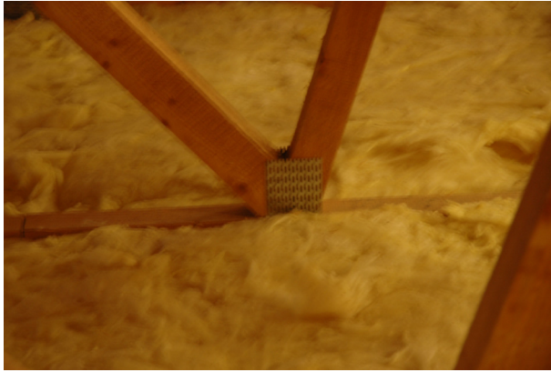
Fig.18 Bad realization of gangnail connection – thin sheet and bad position of the gangnail
