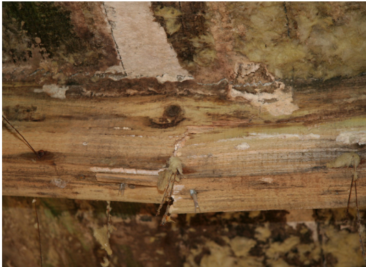
Fig.14 Broken timber beam because of the biological corrosion
