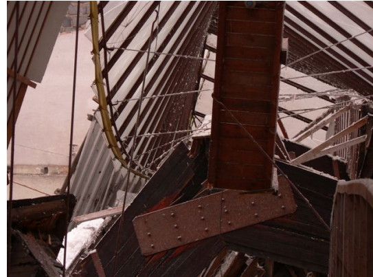
Fig.13 Destroyed roof after the fall down
