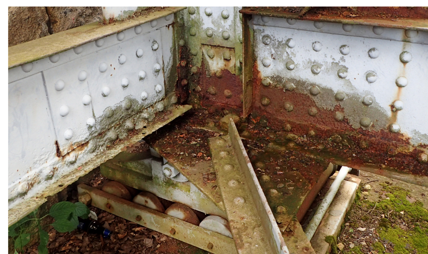
Corrosion damage above abutment
