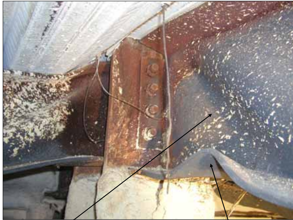
Beam shear buckling
