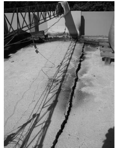
Fig. 6 Crack above intermediate beam first test
