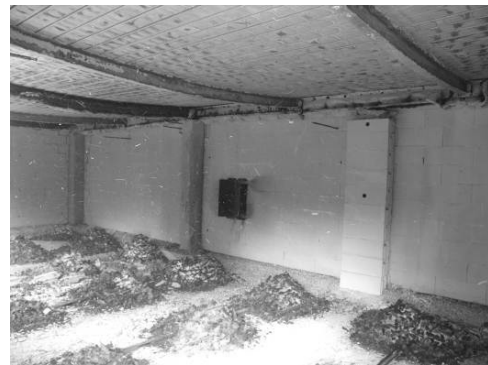
Fig. 2 Second Munich fire test
