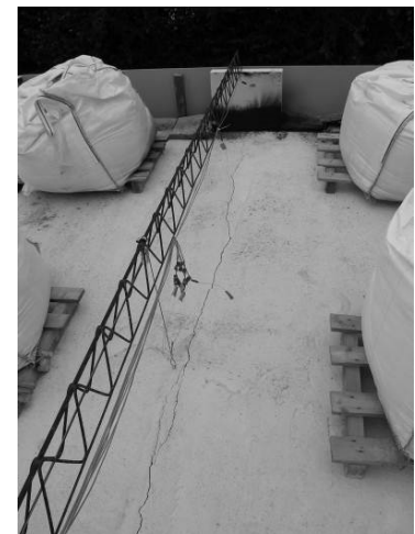
Fig. 8 Crack above intermediate beam second test
