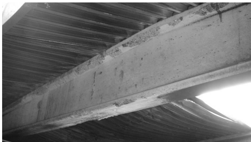
Fig. 3 Fire damage of roof girder
