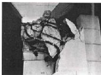
Fig. 1. Large drift and shear failure of a column due to thermal expansion of floor [2]
