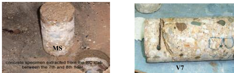
Fig. 5. Change of concrete colour and deterioration of surface layers of specimens
