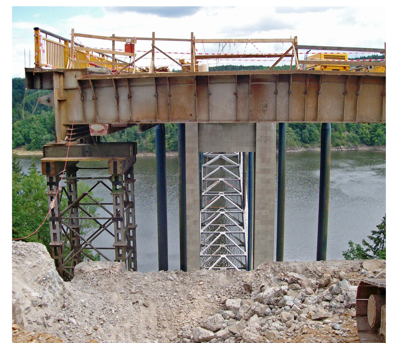
End crossbeam before reconstruction
