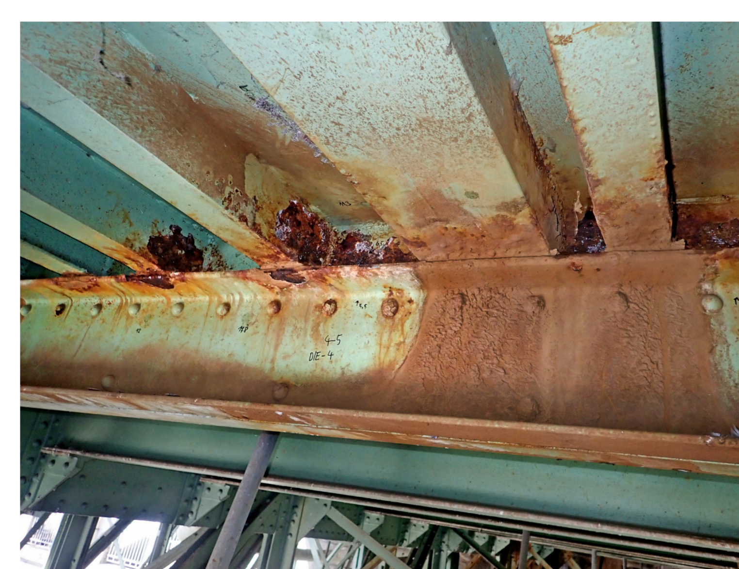
Cracks in bridge deck welds, leakage and leaching of dirt
