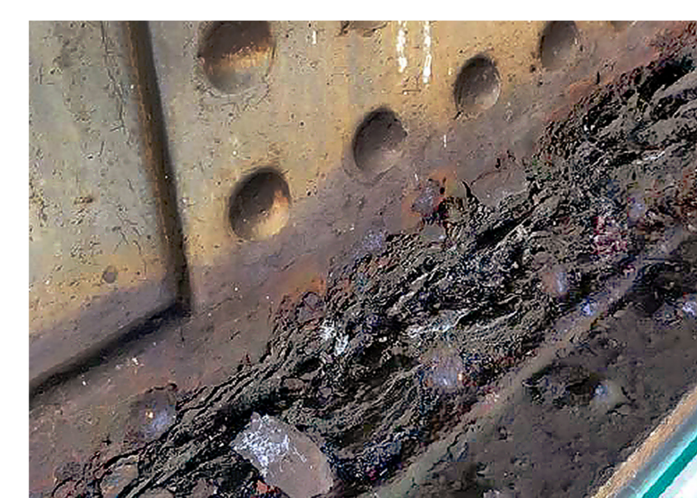
Bottom chord corrosion
