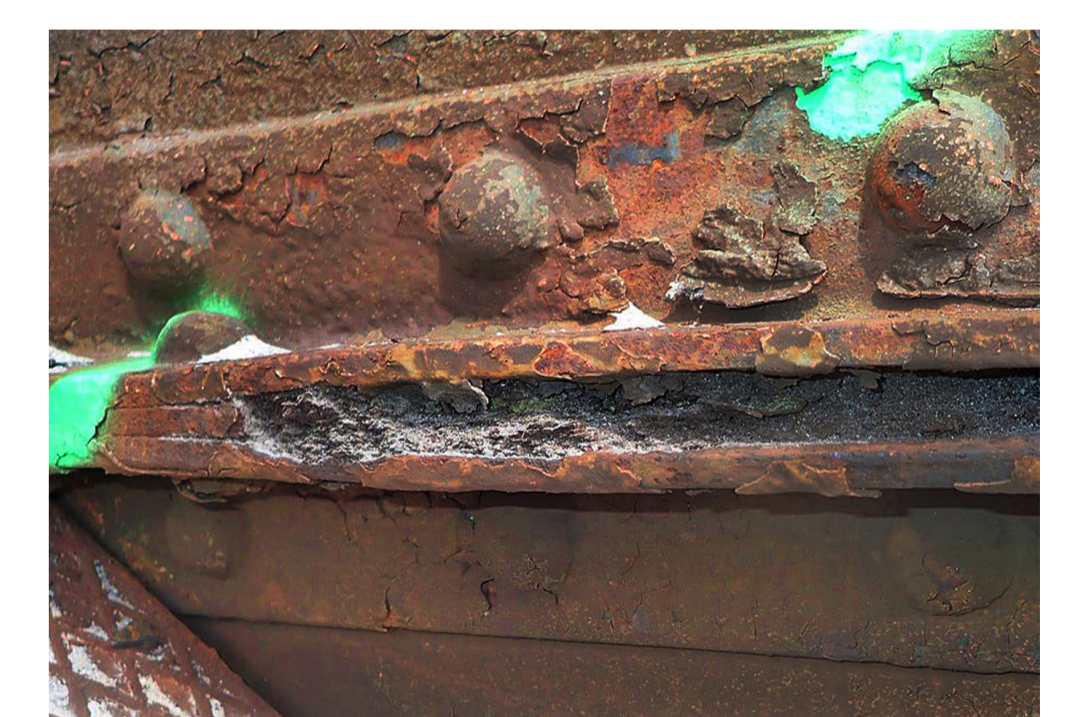
Gap between plates
