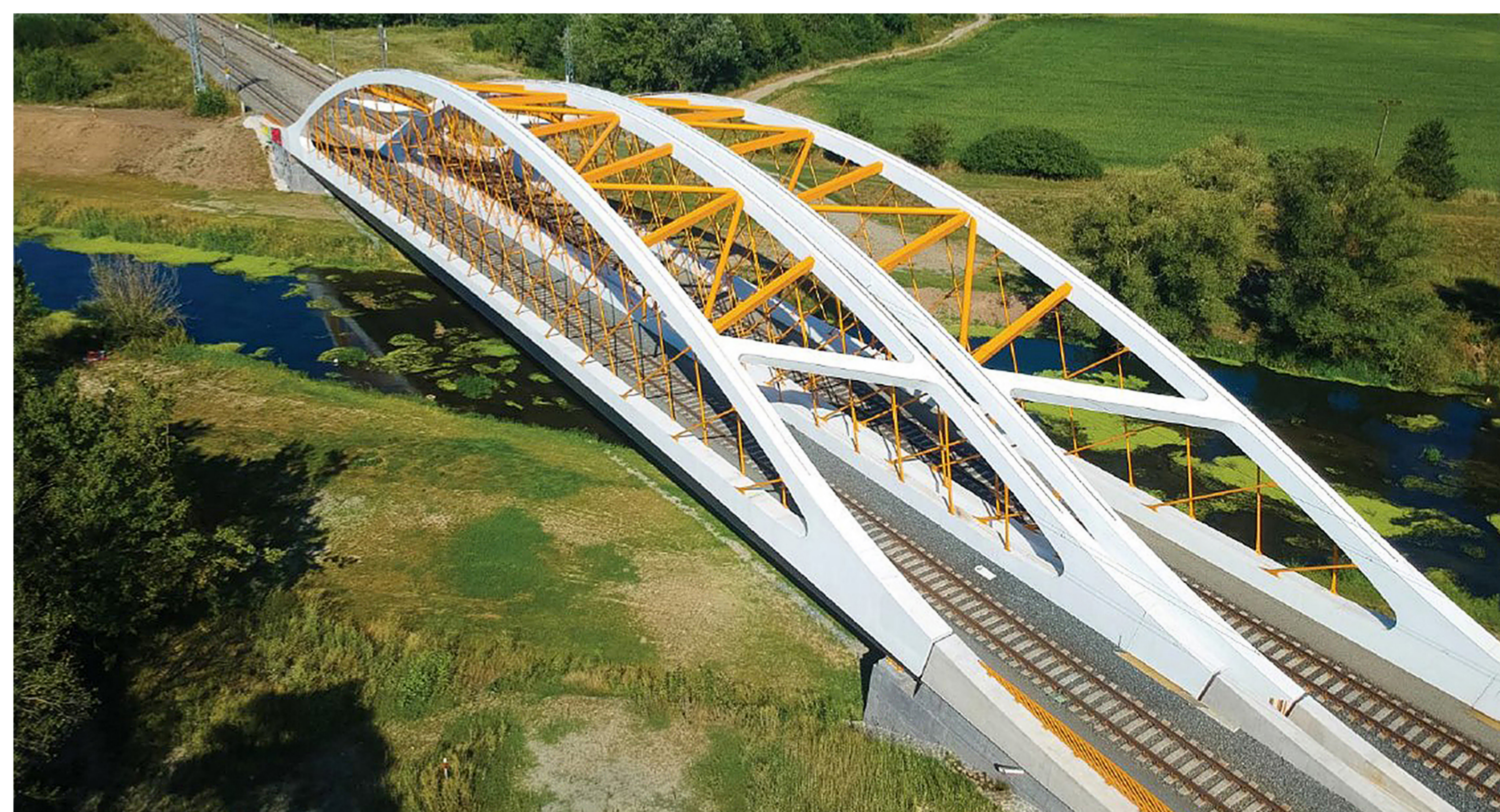
Protection of the Railway bridge over the River Dyje on the Hohenau-Přerov line by duplex coating system, 2016, photo by David Rose
