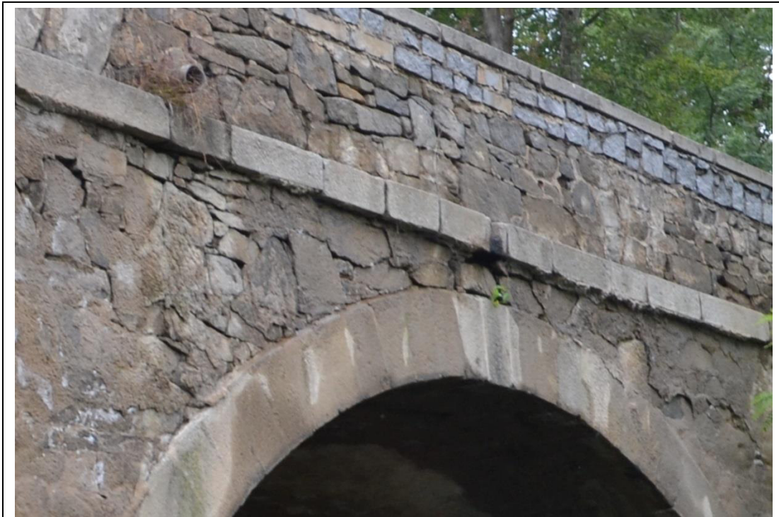
Fig. 11 Horizontal fracture of the spandrel wall over span 2 (upstream side)
