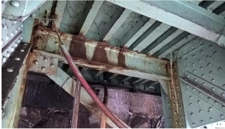
Figure 2.5.3 Liquid seepage through the deck
