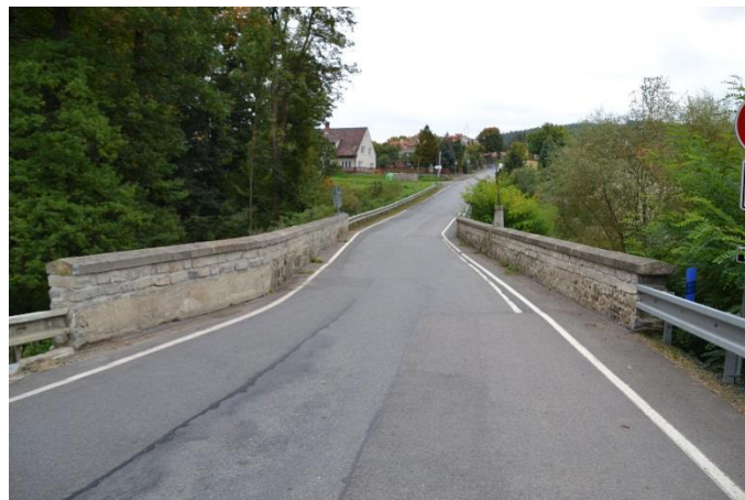
Fig. 3 A view along the road from the left side of the bridge
