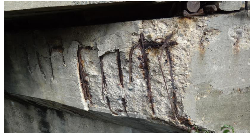
Corrosion of reinforcement on the abutment cap
