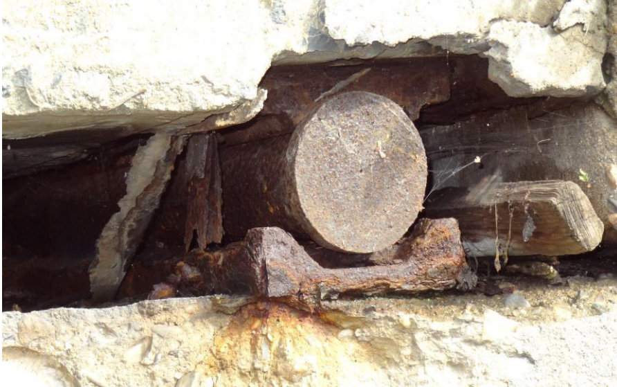
Bearing for longitudinal movement
