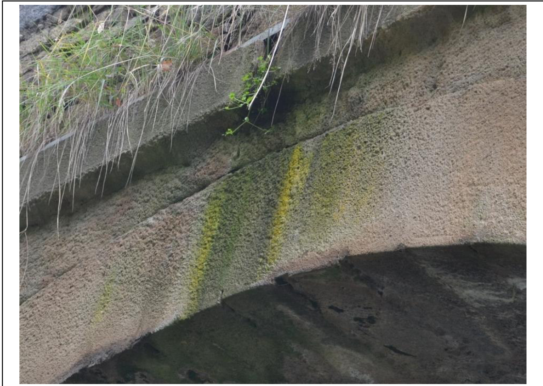
Fig. 17 Leaching in the spandrel wall and parapets in span 2 (downstream side)
