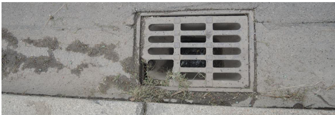
Figure 2.2-13 - Pavement drain - damage on the left is causing the water penetration in the structure
