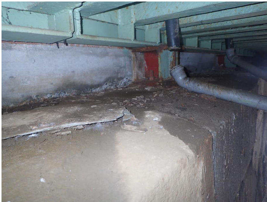
Figure 2.6.2 Disconnected and missing elements
