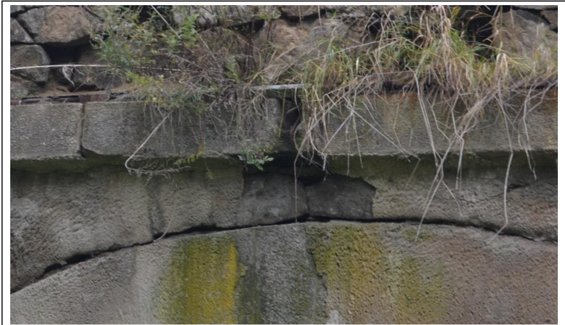
Fig. 13 Horizontal fracture between spandrel wall and the arch over span 1 (downstream side)
