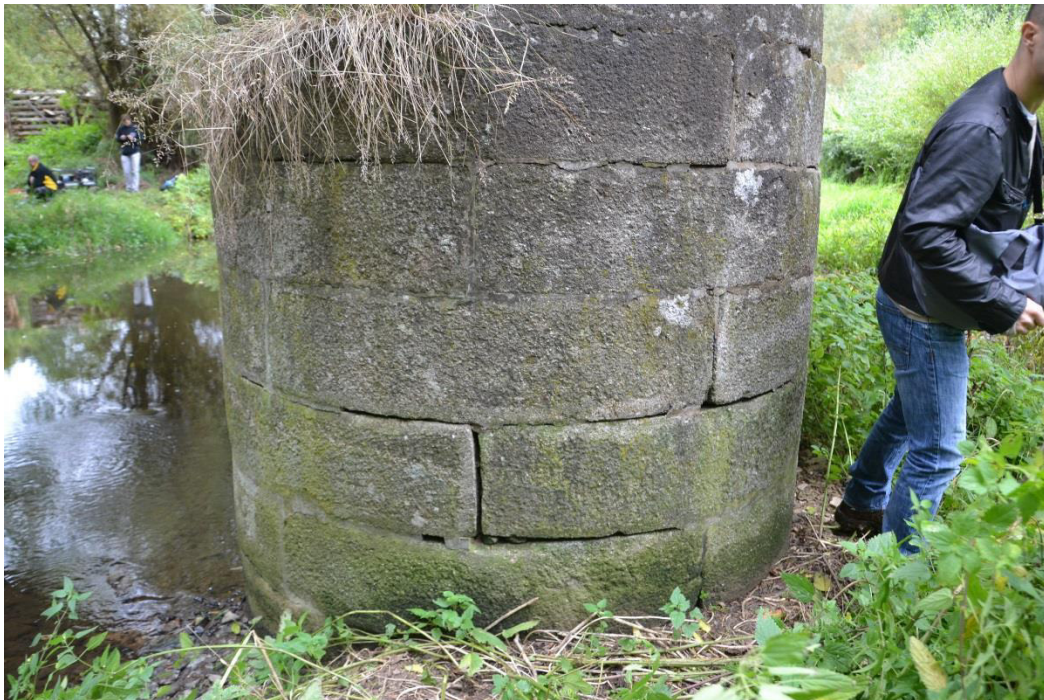
Fig. 21 Loss of mortar in the pier (downstream side)
