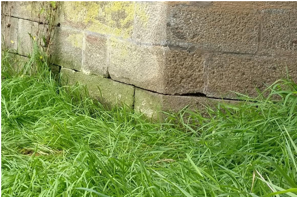
Fig. 22 Loss of mortar in the abutment 1 (upstream side)
