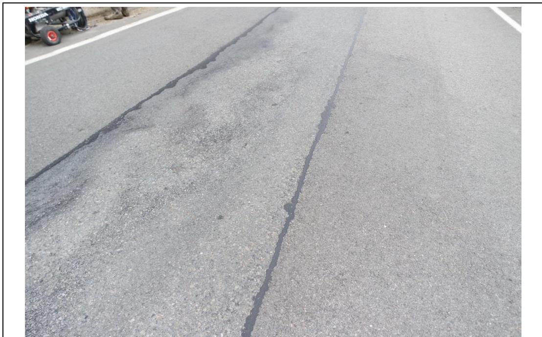
Fig. 28 Cracks and shoving of the pavement
