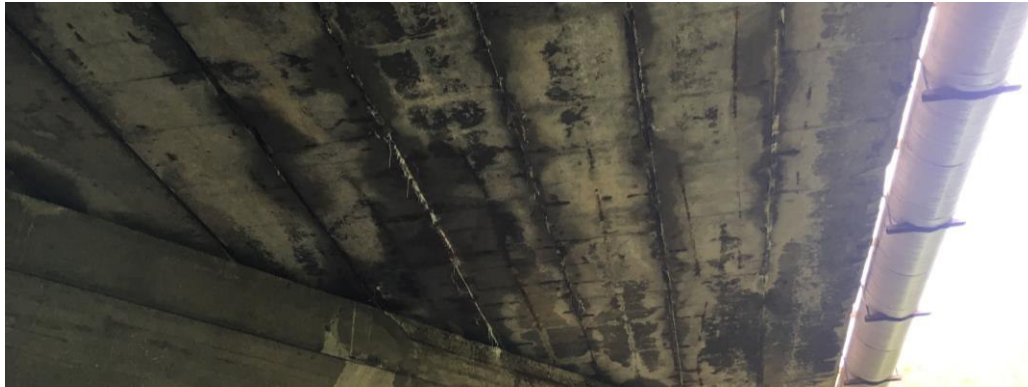
Figure 2.2-6 - Initiation of longitudinal reinforcement corrosion on girders G1-G5
