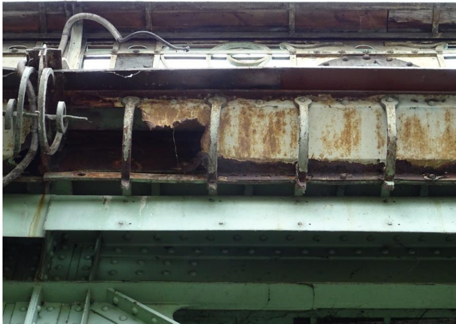
Figure 2.14.1 Corroded edge plates and loss of section
