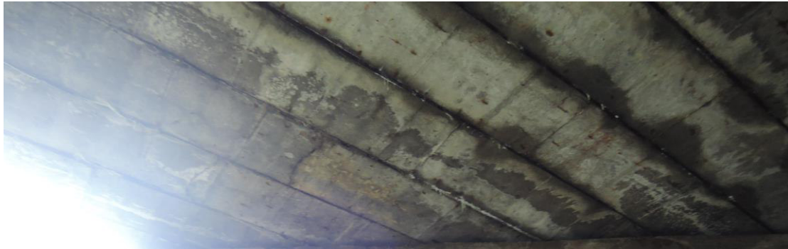
Figure 2.2-3 - Leakage between girder joints
