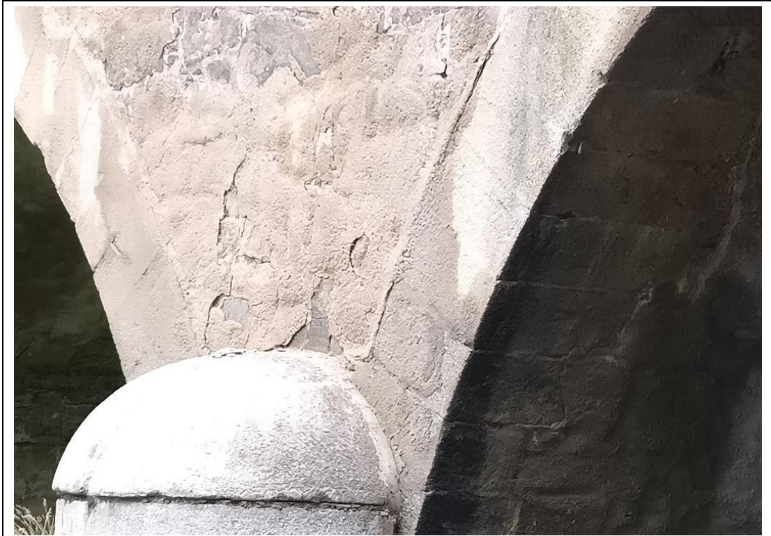
Fig. 14 Horizontal fracture of the spandrel wall over the pier (upstream side)
