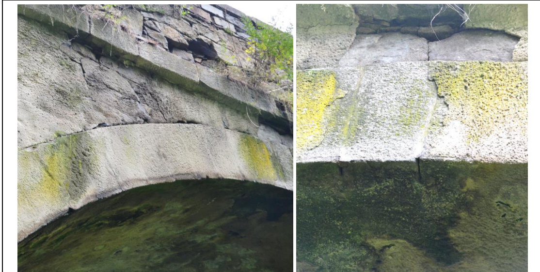
Fig. 16 Leaching in the spandrel wall and parapets in span 1 (downstream side)
