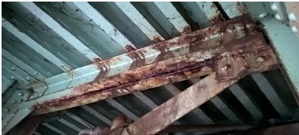
Figure. 2.3.2 Mild surface corrosion observed
