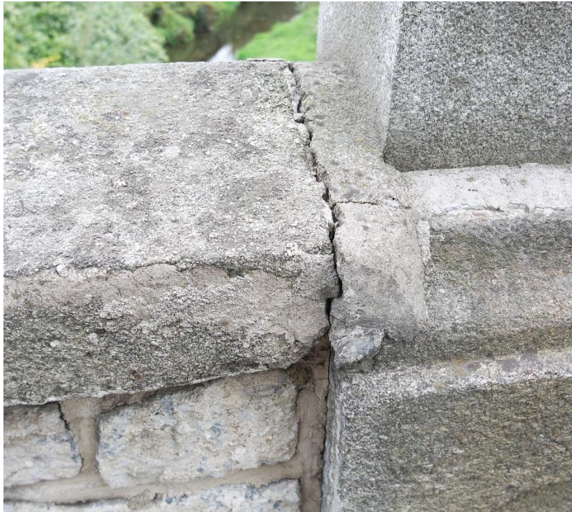
Fig. 26 Transverse cracking of parapet (upstream side)
