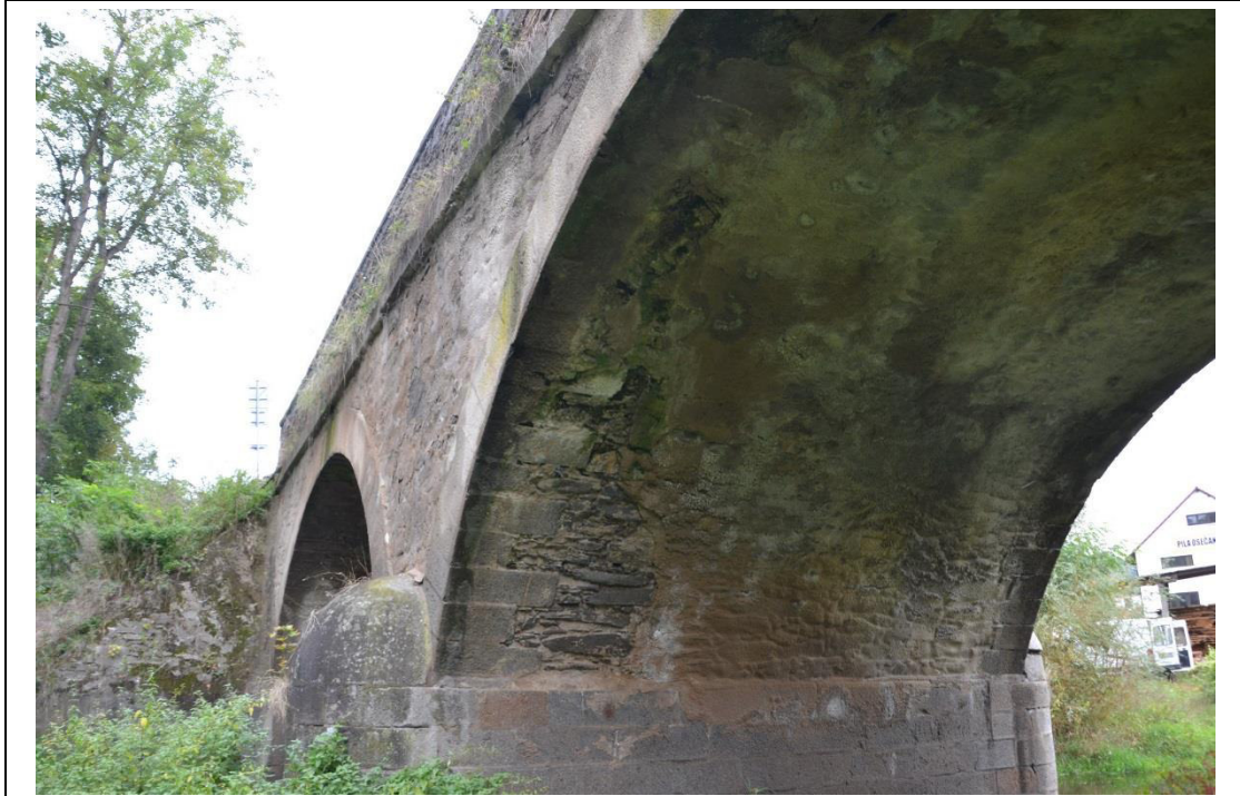
Fig. 15 Leaching in the arch in span 1
