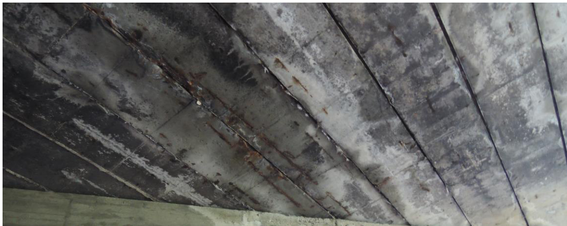
Figure 2.2-7 - Initiation of longitudinal reinforcement corrosion on girders G1-G7
