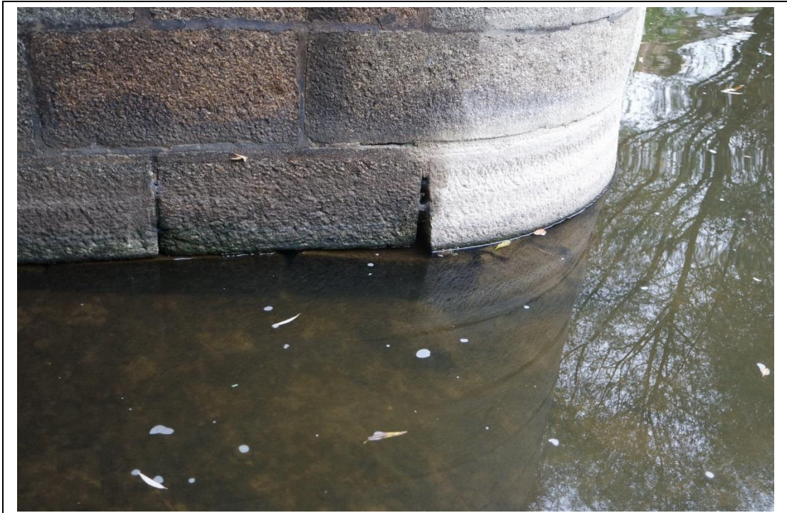
Fig. 9 Scour of the pier (upstream side)
