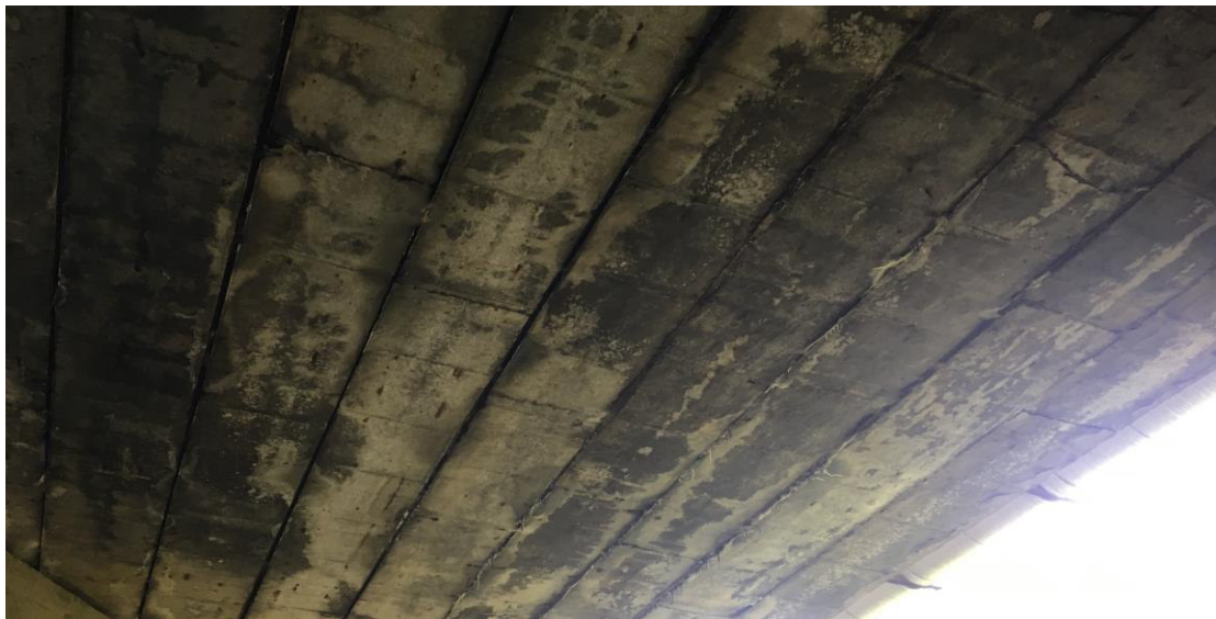
Figure 2.2-2 - Leakage between girders joints
