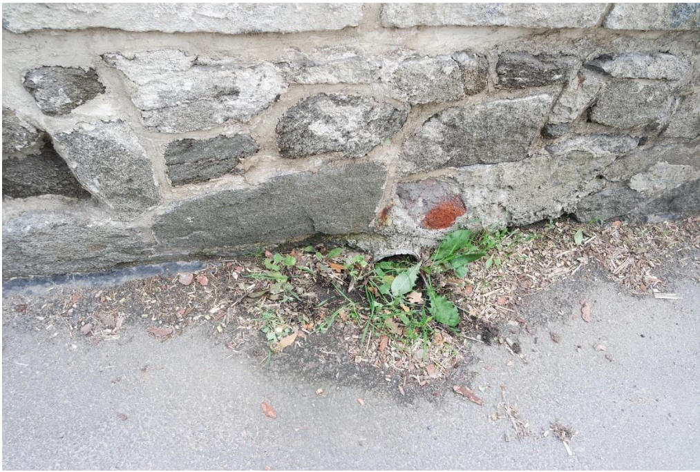
Fig. 25 Degradation of stones in parapet (upstream side)
