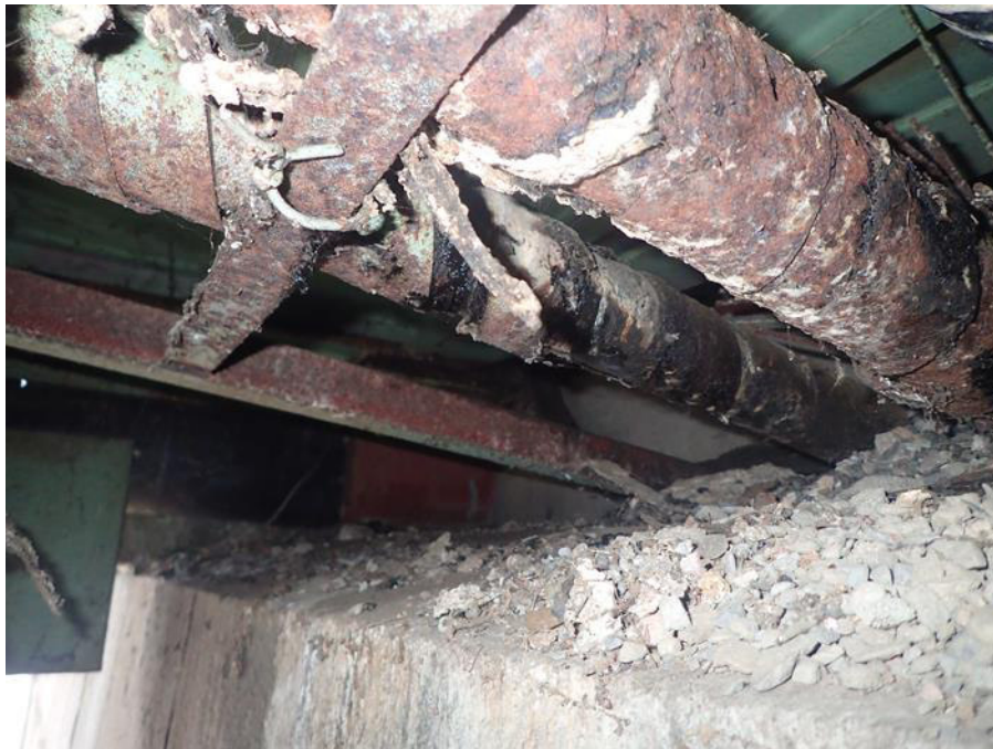
Figure 2.13.1 Corroded communications pipes
