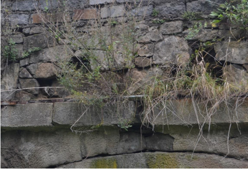
Fig. 23 Loss of blocks in parapet (downstream side)
