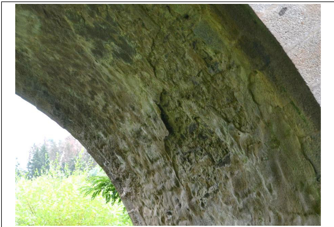
Fig. 18 Leaching in the arch in span 1
