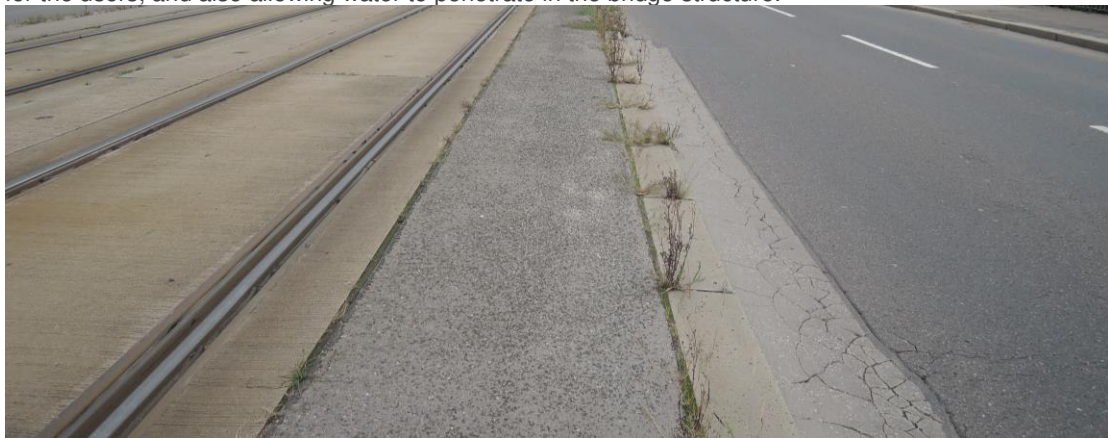
Figure 2.2-12 - Cracks and vegetation in the middle strip
