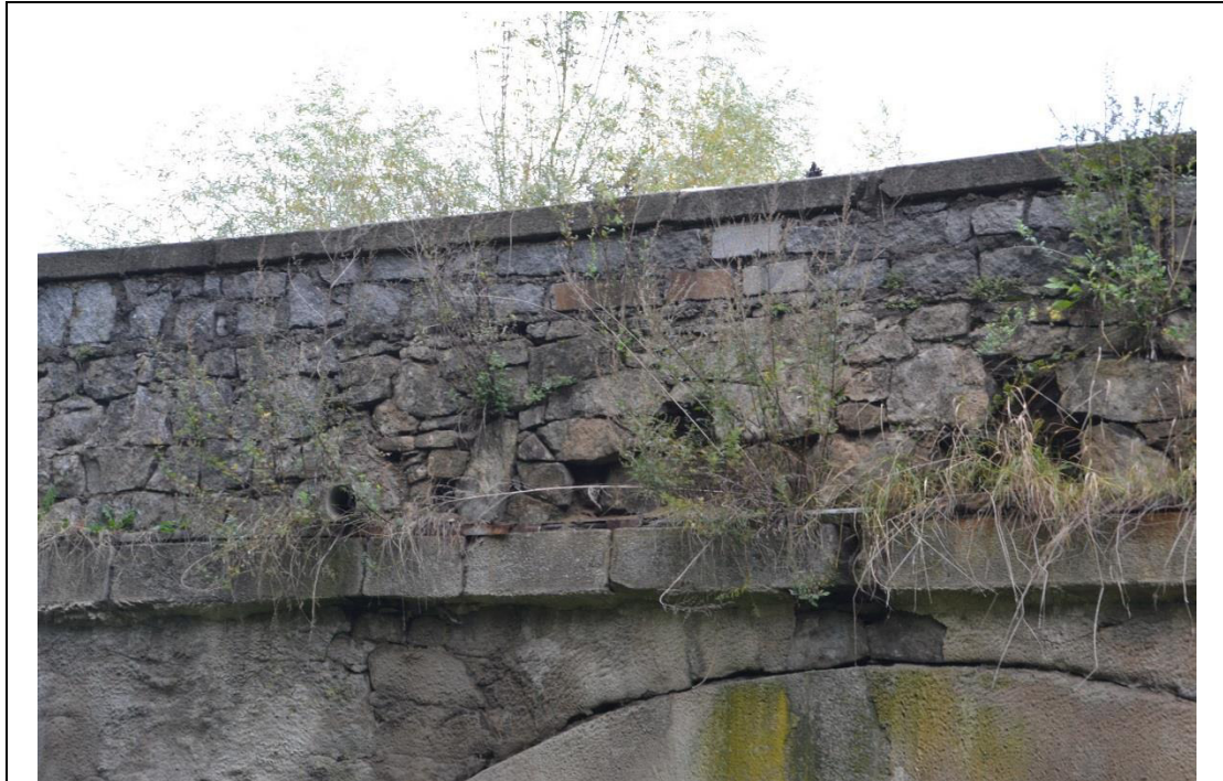
Fig. 31 Improperly shaped drainage pipes (downstream side)
