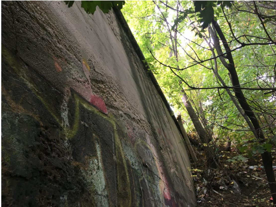
Figure 2.1-16 – Loss of cement matrix at wingwall
