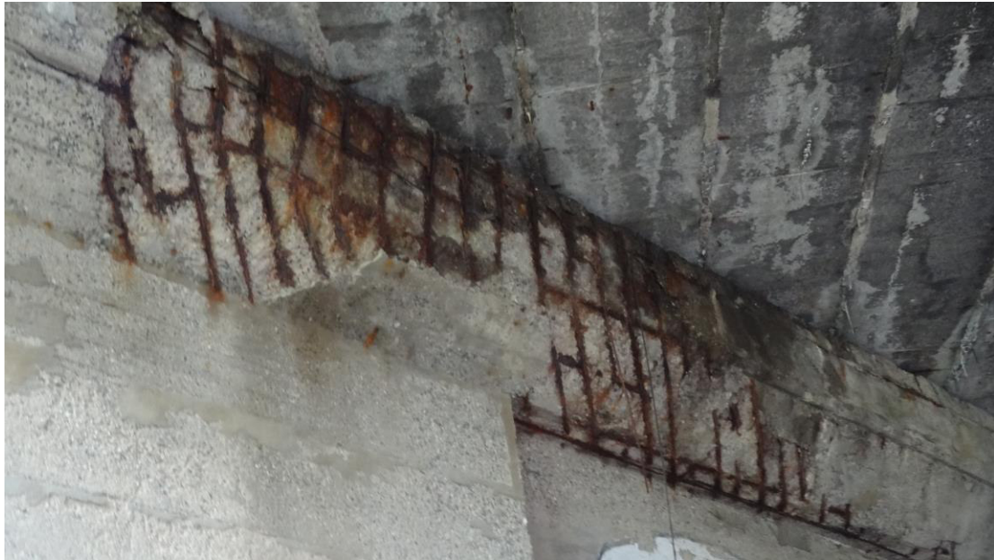
Figure 2.1-8 - A2-1 damages of concrete cover and corroded bars
