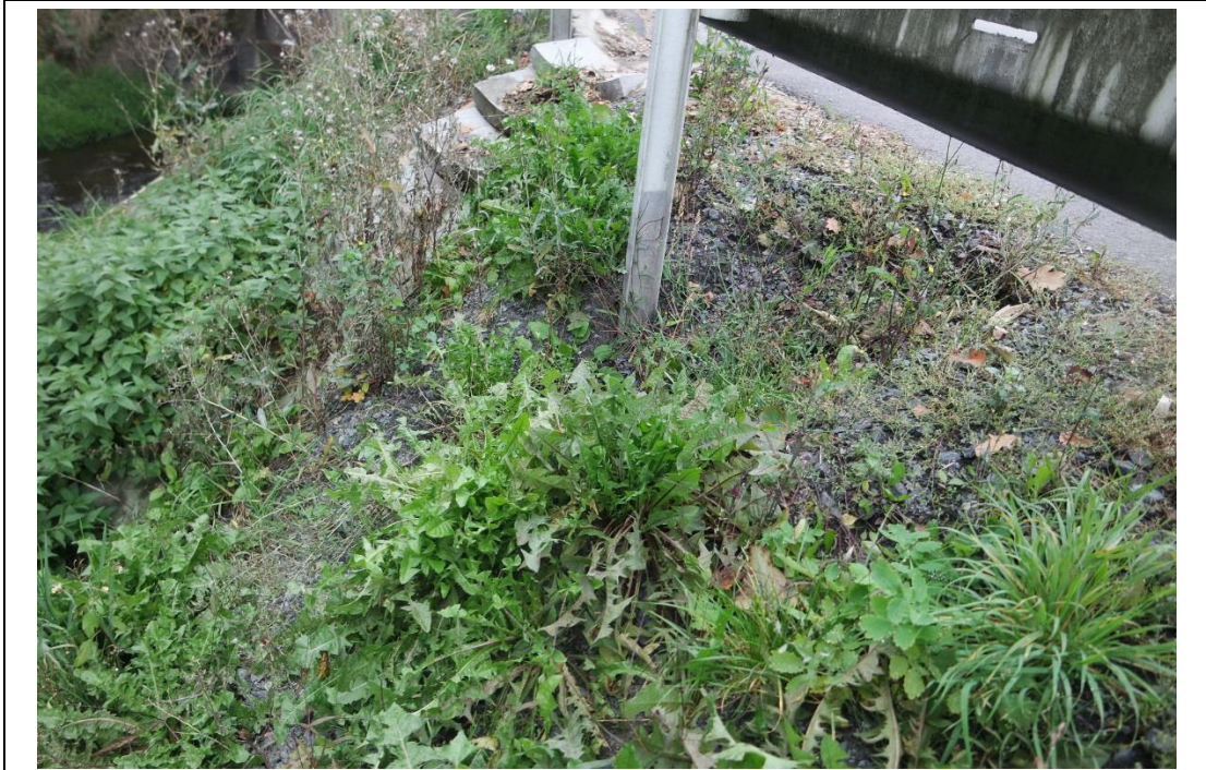
Fig. 29 Erosion of the embankment over abutment 1 (downstream side)
