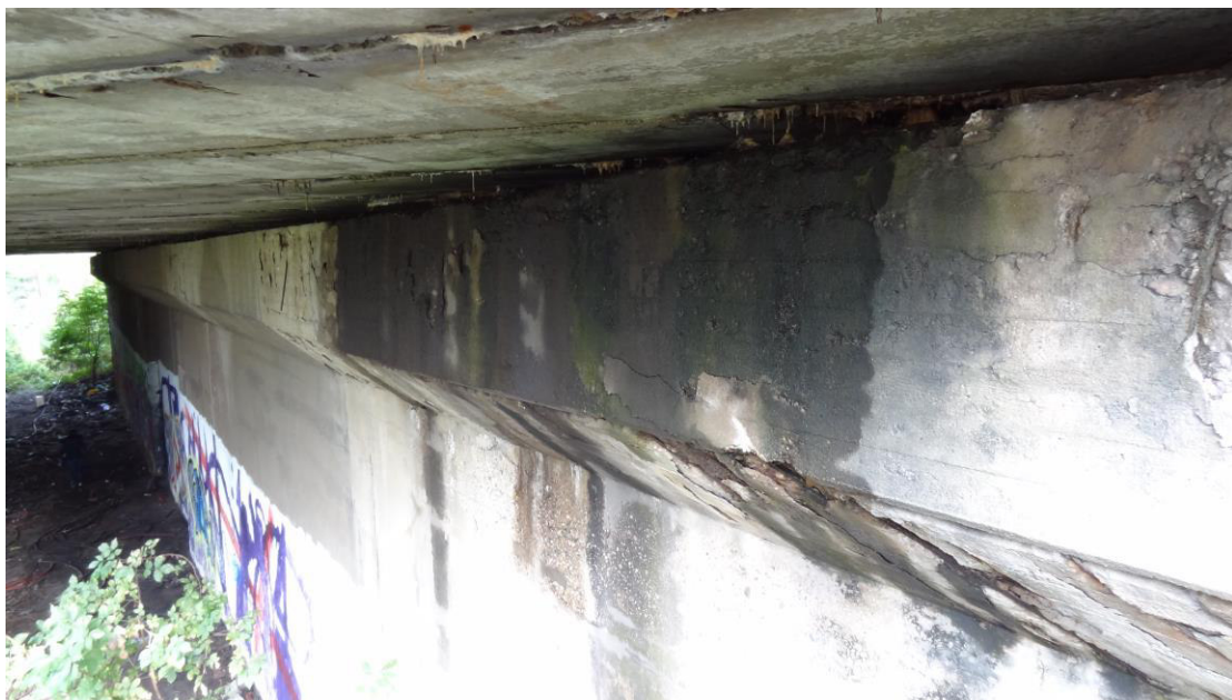
Figure 2.1-9 – Water leakage at A1-3
