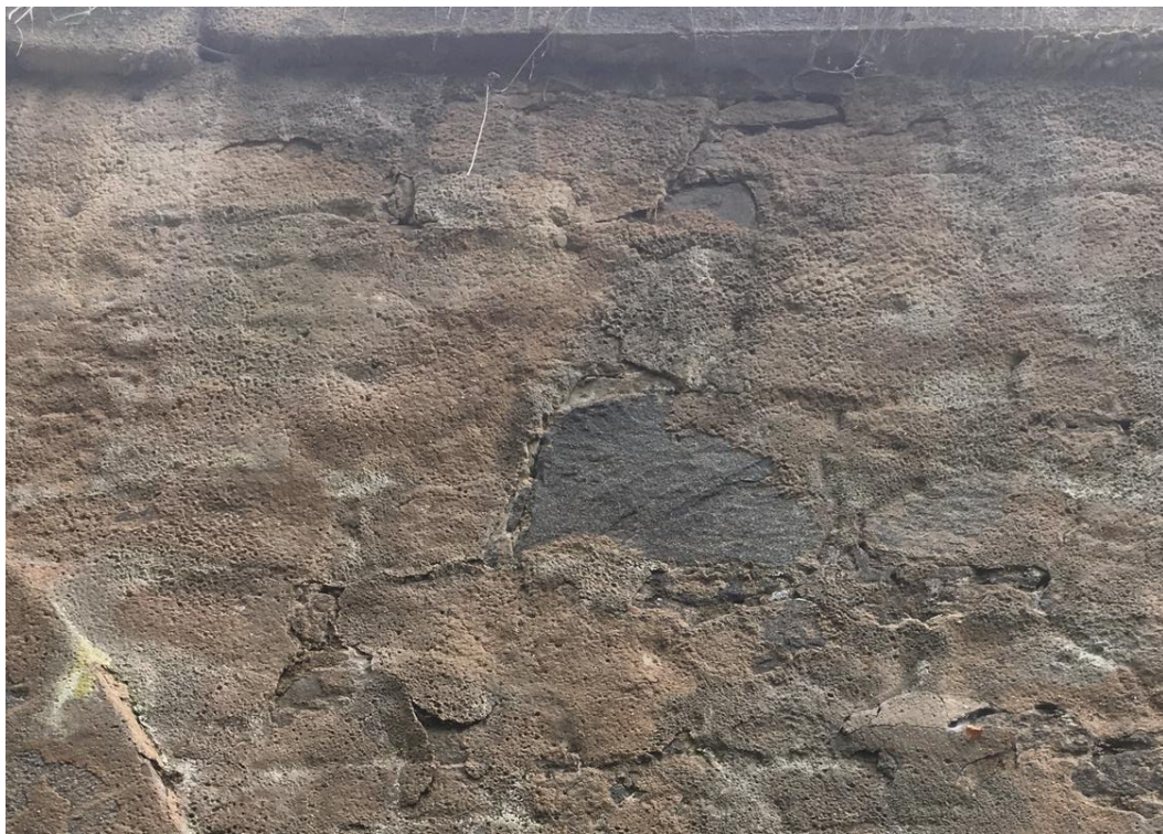
Fig. 12 Vertical fracture of the spandrel wall over pier (downstream side)
