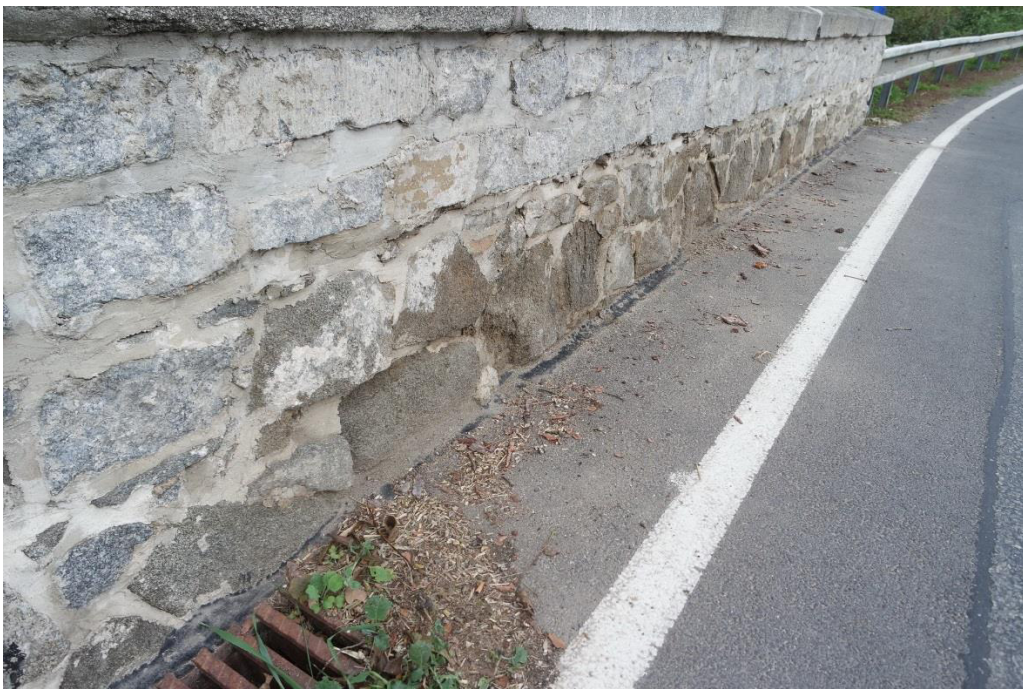
Fig. 24 Degradation of stones in parapet (downstream side)
