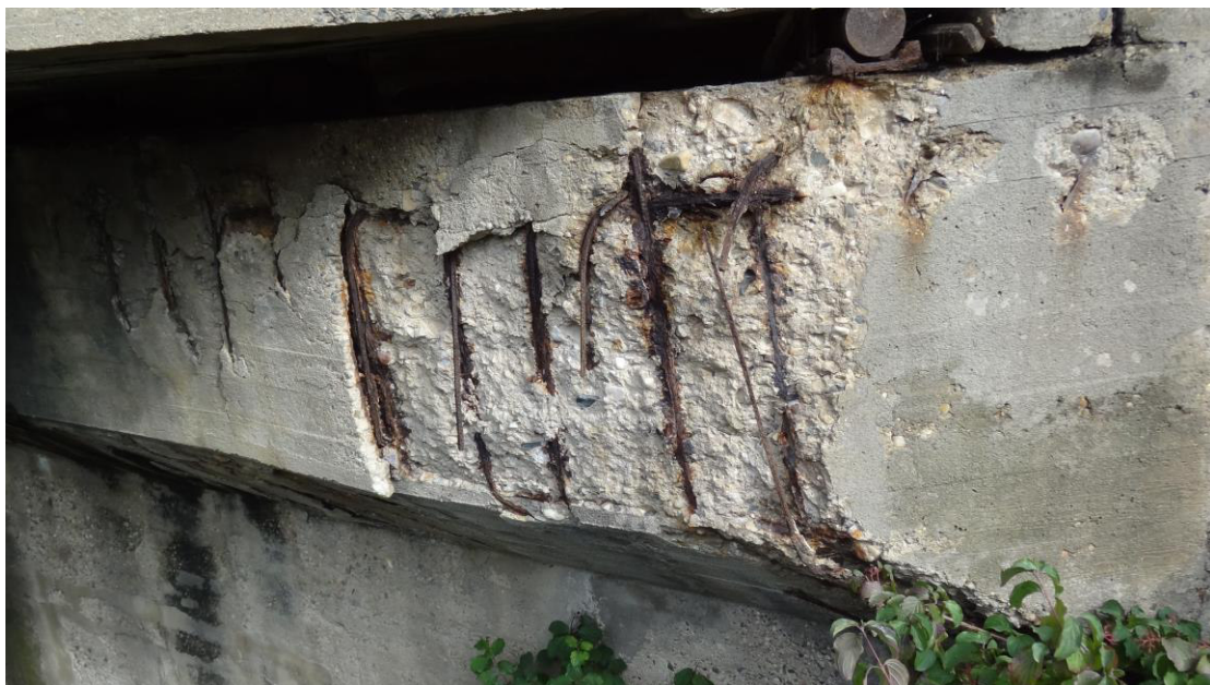
Figure 2.1-7 – A1-3 damages of concrete cover and corroded bars
