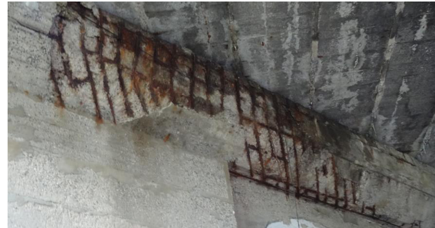
Corrosion of reinforcement on the abutment cap
