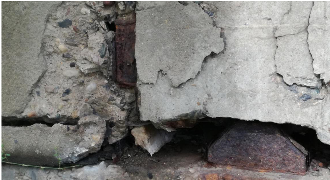
Figure 2.2-10 - Corrosion of anchorage plate and spalling of surrounding concrete
