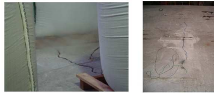
Fig. 20 – State of slab at central part of the floor during and after the test
