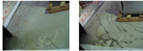
Fig. 19 – State of slab around steel column
