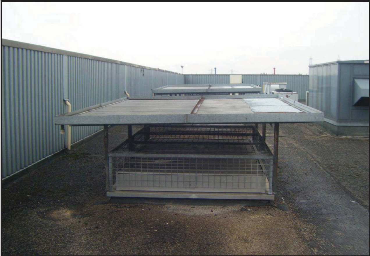
Fig. 13.5 Roof ventilation covers
