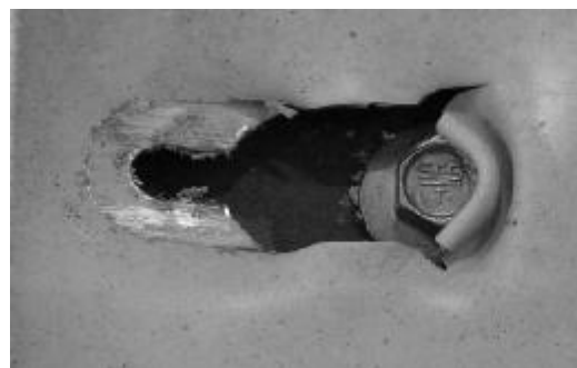
Fig. 9 The collapse mode of the connection from set C, temperature 200°C
