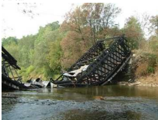
Fig. 1. Bridge collapsed after fire [12]
